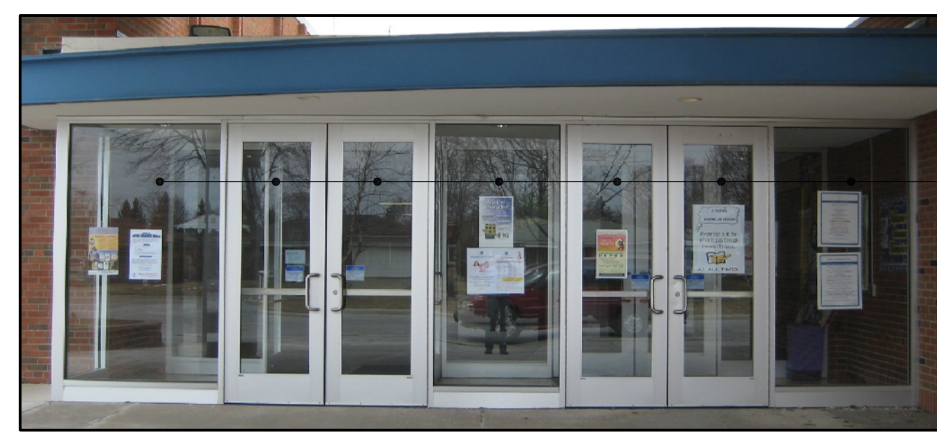
NOTE: PHOTO SHOWN IS EXTERIOR- FILM TO BE INSTALLED AT INTERIOR SIDE OF GLAZING
